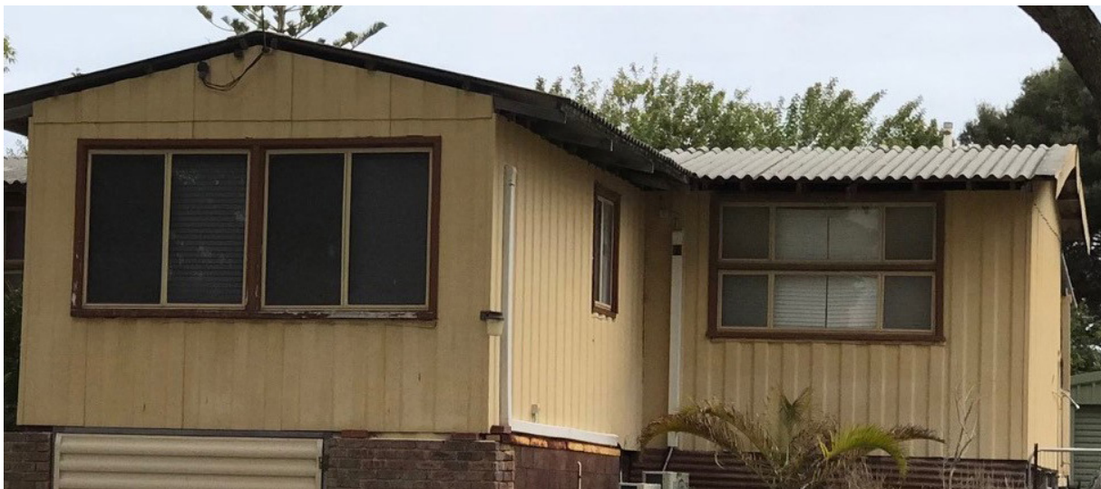
FIGURE 14: Residence with multiple AC structural components
