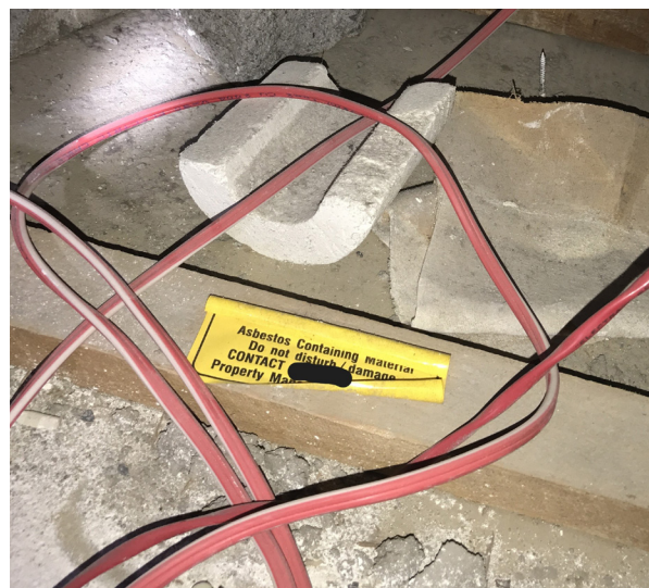
FIGURE 9: Section of thermal pipe insulation located in ceiling space, with debris
