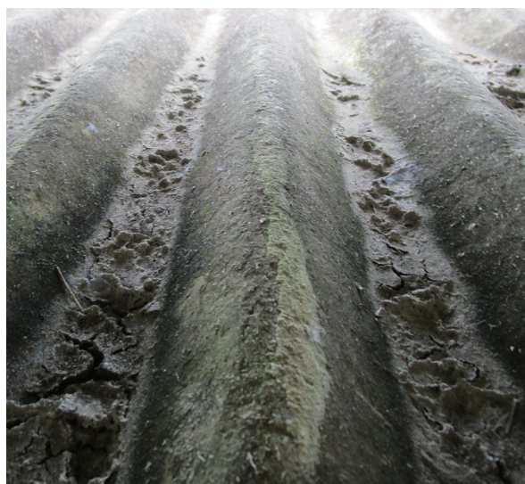
FIGURE 13: AC dust/debris on AC corrugated roof with organic growth
