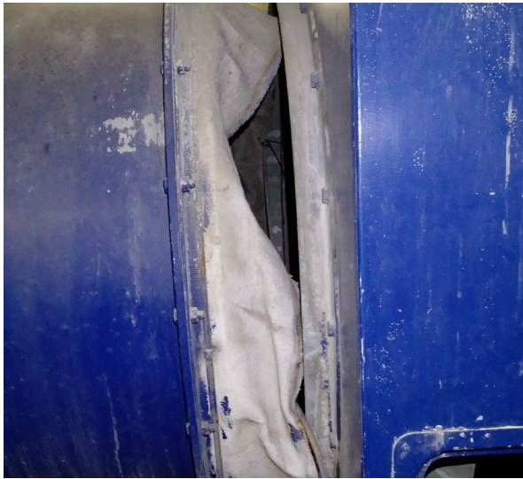
FIGURE 4: Woven asbestos flexible duct seal on vibration isolator
