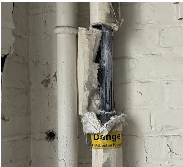
FIGURE 6: Damaged asbestos insulation to pipe
