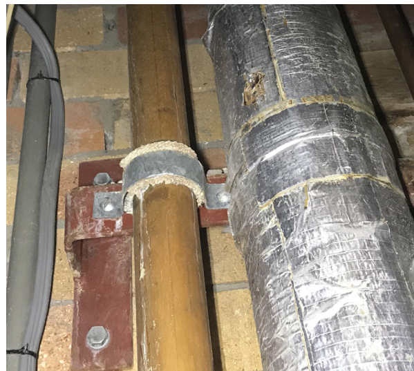
FIGURE 7: Woven asbestos textile under pipe bracket in service riser
