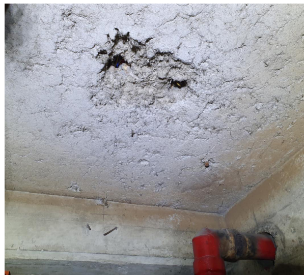
FIGURE 17: Damaged sprayed coating which was originally tamped
