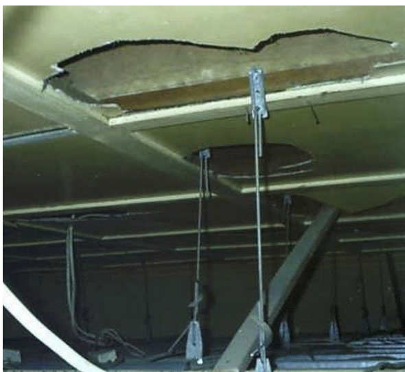
FIGURE 8: Original asbestos cement ceiling damaged when suspended ceiling system installed
