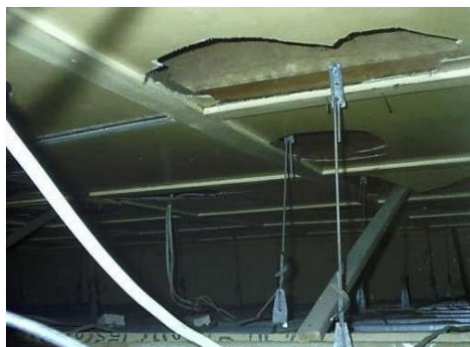
Figure 8: Original asbestos cement ceiling damaged when suspended ceiling system installed
