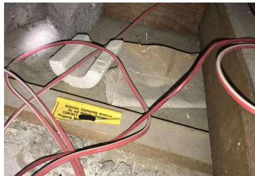
Figure 9: Section of thermoplastic pipe insulation located in ceiling space, with debris.
