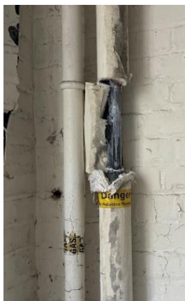
Figure 6: Damaged asbestos insulation to pipe
