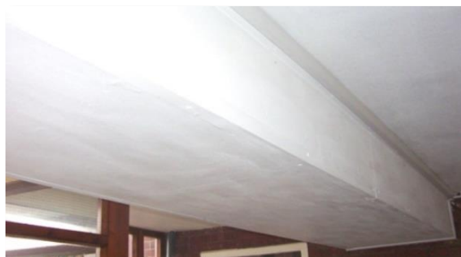
Figure 15: Airconditioning duct clad in low density fibreboard sheeting
