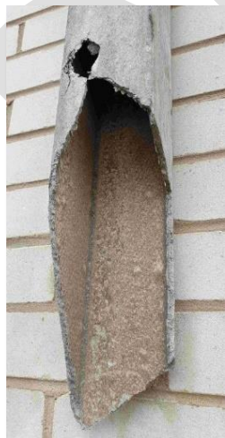
Figure 10: Damaged AC downpipe
