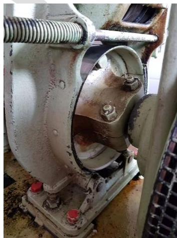
Figure 5: Brake pads on lift motor
