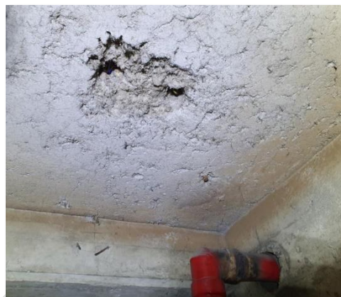
Figure 17: Damaged sprayed coating which was originally tamped
