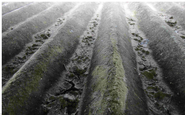
Figure 13: AC dust/debris on AC corrugated roof with organic growth
