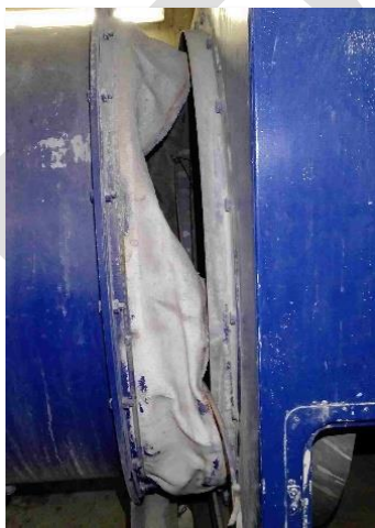
Figure 4: Woven asbestos flexible duct seal on vibration isolator
