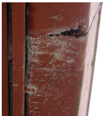
Figure 12: AC debris under roof guttering from AC roof
